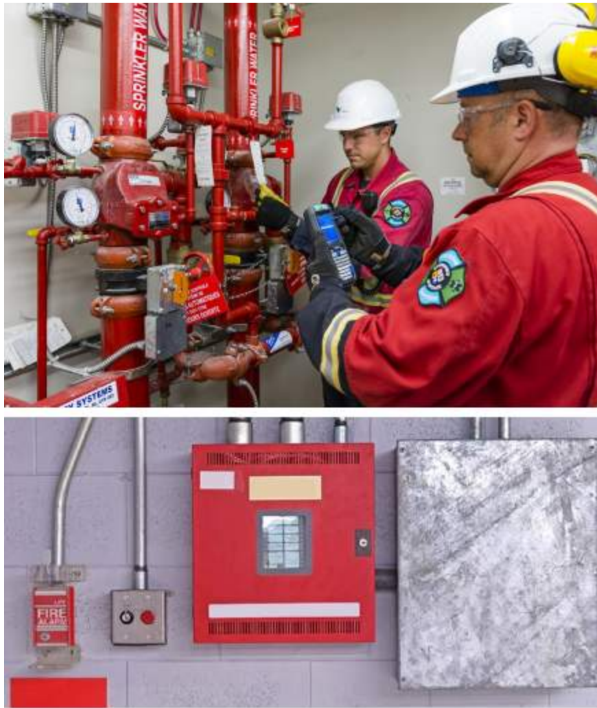
Sprinkler System / Fire Detection System
